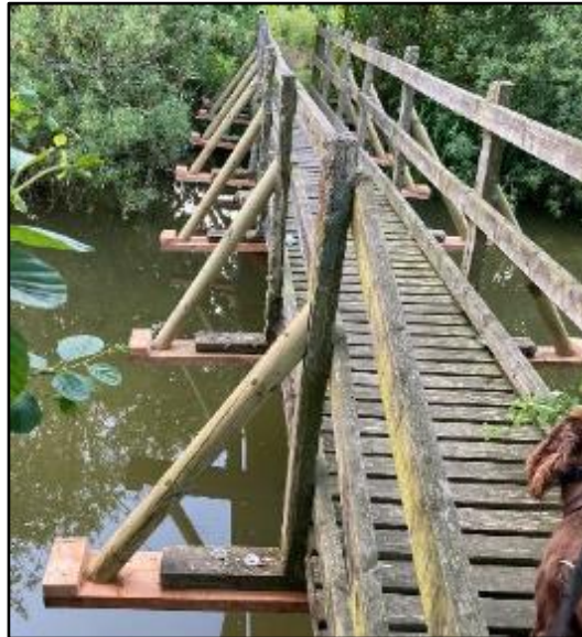
Above: Rotten timbers replaced by the Midmar Men's Shed on a bridge at the local Stillwater Fishery
