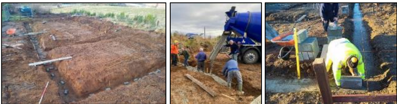
Perimeter foundation dug (left), Concrete is poured (centre), and the First Block is laid (right)
